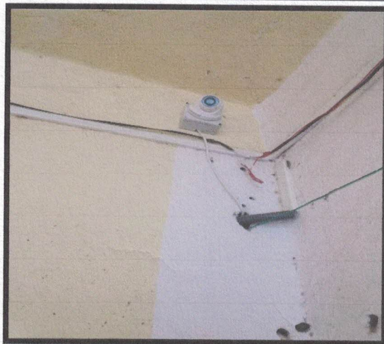
CCTV Surveillance in campus
