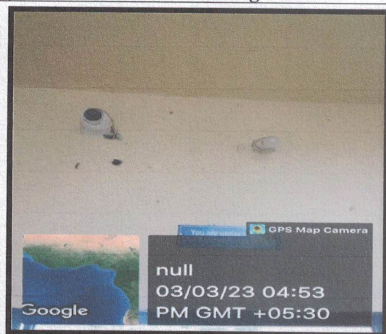
CCTV Surveillance in campus
